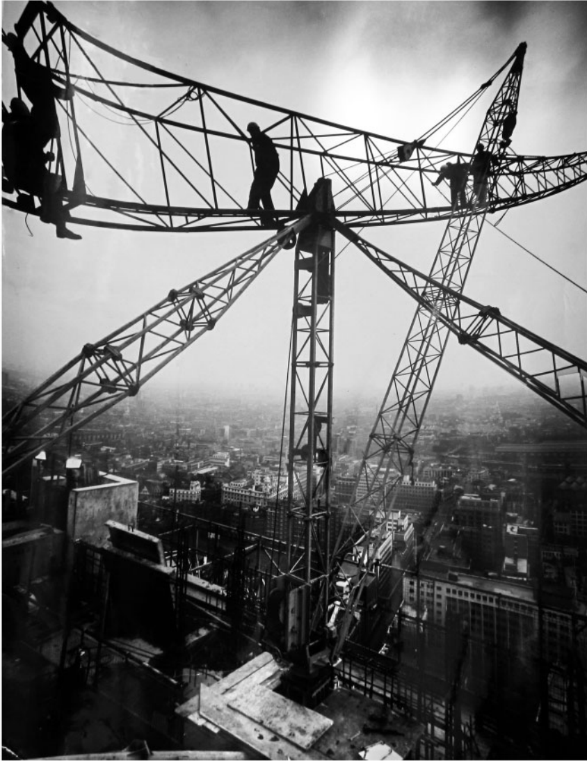
Fig. 1. Crane erectors on Laing Barbican site. Photograph by John Steeden, reproduced with his permission.
